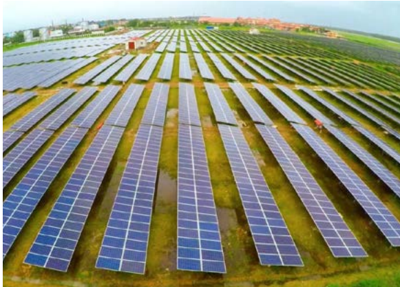
Figure 10.1: Aerial view of the solar PV project Source: Bosch Building Solutions ( https://www.boschbuildingsolutions.com/x/en/news-and-stories/cochin-international-airport-india/ )
